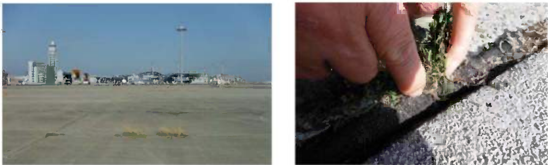
Fig. 4. Weed invasion to concrete pavement in airport apron
